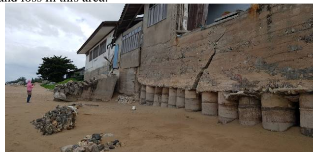
Fig. 7. Beach erosion and property damages along Ban Thung Pradu.
